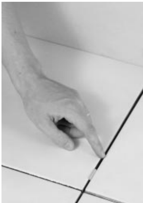
Carve/route grout joint 1/2" deep. Install sensor. Reinstall grout over sensor and sensor wire.
